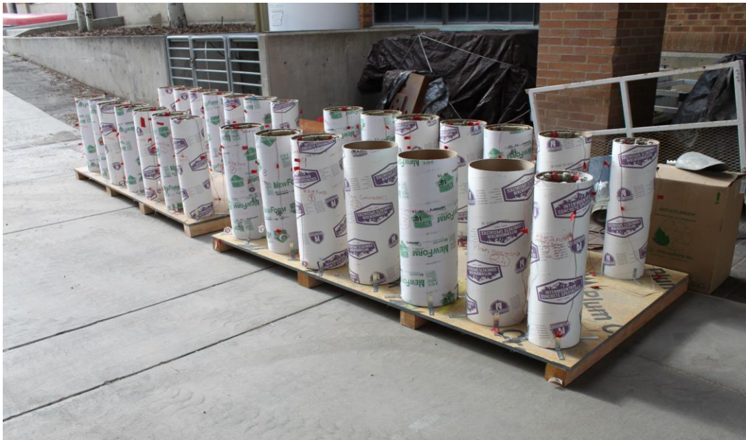
Figure 2.6: GFRP cages placed in sonotubes and fixed on wooden planks with steel brackets.
