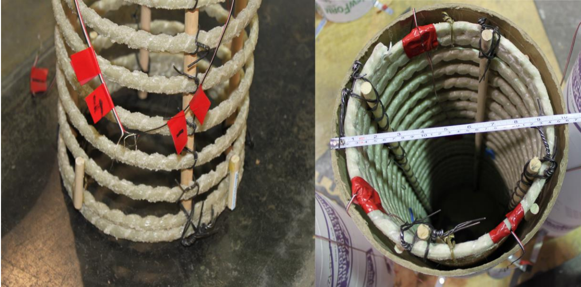
Figure 2.5: Wooden dowels used to maintain clear cover of concrete and pitch of the spiral.
