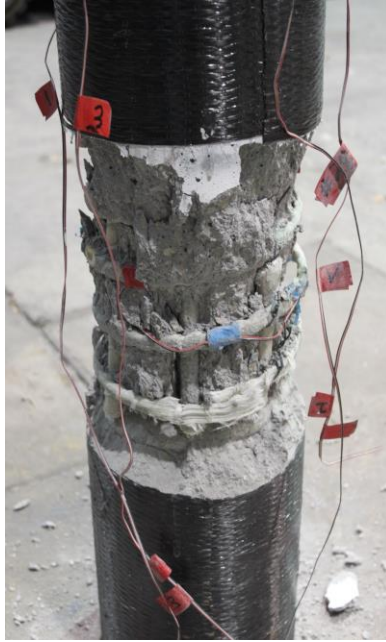
Figure 3.11: GFRP reinforced concrete column 6LR#3@1.5 at failure.
