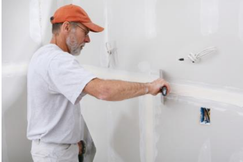
Figure 6. Worker applying joint compound. Adapted from “Craftsman Finishing Drywall Joint,” by Earley Construction, 2009. Retrieved from http://homebuilderjacksonville.com/wp-content/uploads/2009/10/drywall-repair-and-installation-in-jacksonville-nassau-county-orange-park-middleburg.jpg Copyright 2009 by Earley Construction.
