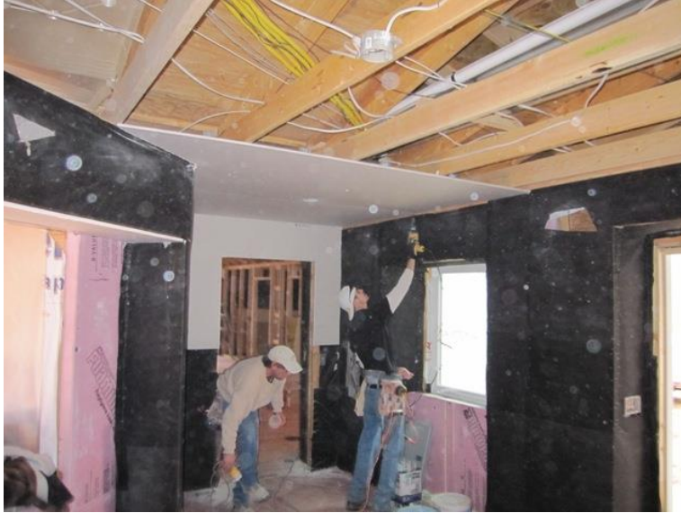
Figure 4. Worker fitting and installing drywall in residential building. Retrieved from http://www.brainright.com/OurHouse/Construction/Drywall/20091124004_Installing%20drywall.jpg . Copyright n.d. by Jay McClellan.
