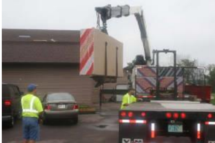
Figure 2. Delivery of drywall to jobsite. Humane Society. Retrieved from http://cchs-petshelter.org/sitebuildercontent/sitebuilderpictures/.pond/Aug28c.jpg.w300h200.jpg Copyright 2016 by Clark County Humane Society.
