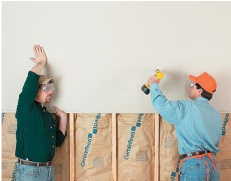
Figure 5. Workers attaching drywall to framing. Adapted from “How to hang basement drywall,” by stepbystep.com, n.d. Retrieved from http://www.stepbystep.com/wp-content/uploads/2013/01/How-to-Hang-Basement-Drywall1.jpg . Copyright 2016 by Stepbystep.com
