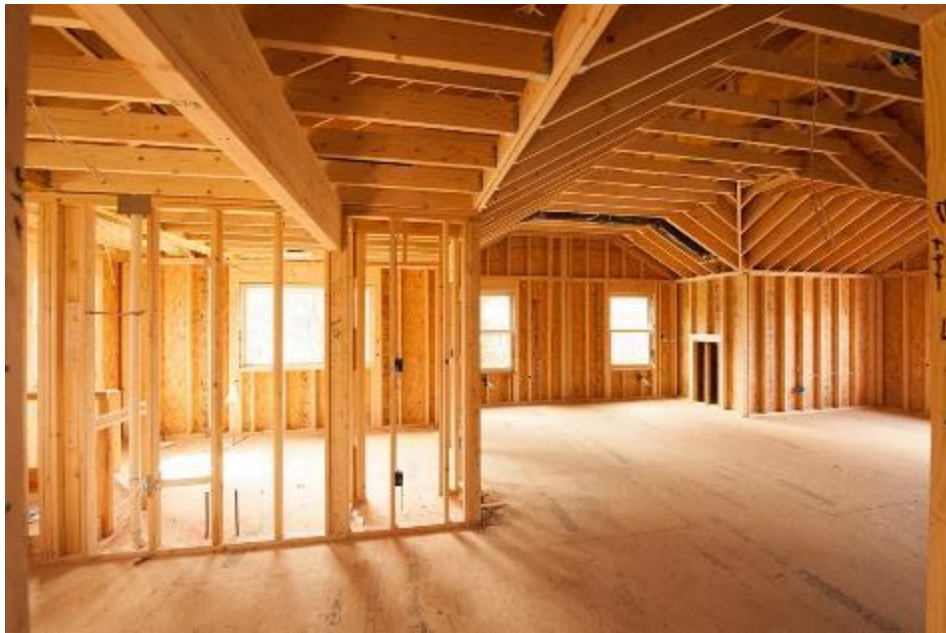
Figure 1. Framing of a house ready for drywall installation. Adapted from “CotY 2013 Award: Entire House, Framed House Structure,” by EDW Builders, 2013. Retrieved from http://www.edwbuilders.com/wp-content/uploads/2013/02/EDW_Builders_CotY_2013_Entire_House_Framing_2.jpg . Copyright 2013 by Bob Graham, Jr. Photography.
