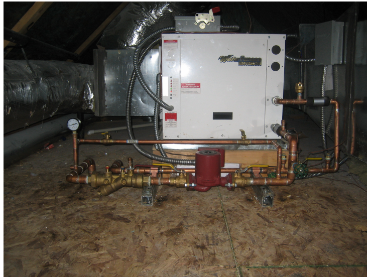
Figure 2.33: Heat Pump and Inline Pump. The heat pump and inline pump were installed in the attic above the second floor. The heat pump is the large, white device and the inline pump is the small, red device below the heat pump in the figure.
