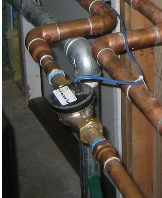
Figure 2.3: Flowmeter. The flowmeter installed in the first floor mechanical room
