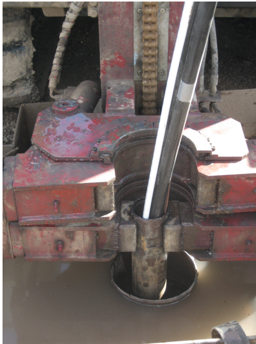
Figure 2.31: U-tube Insertion. The heavily monitored U-tube during installation, showing the U-tube, pex and TCs being inserted into the drill casing.
