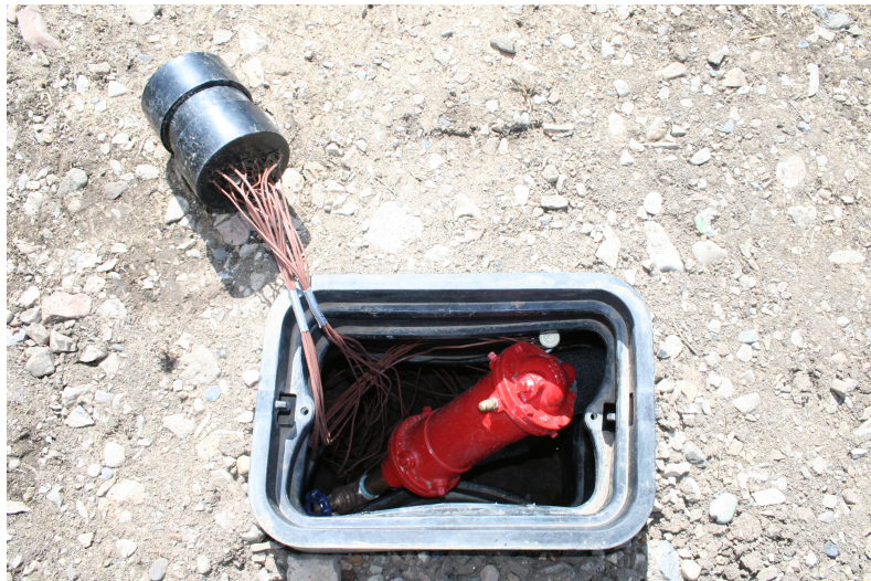
Figure 2.9: Sprinkler Box for H.X.. A sprinkler box providing access to thermosiphon heat exchanger and a thermocouple junction enclosure.
