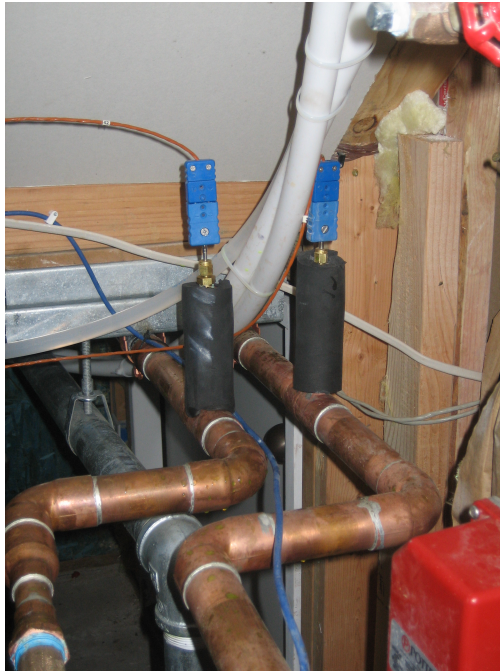
Figure 2.2: Immersed Thermocouples. Immersed thermocouples installed in the first floor mechanical room
