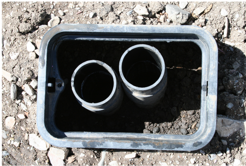
Figure 2.13: Valve Enclosure Access. A sprinkler box with ABS pipes providing access to three-way valves in the buried valve enclosure.
