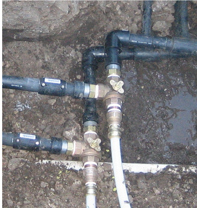
Figure 2.10: Three-way Valves. Three-way valves installed in the propylene glycol supply and return lines for the heat pump.
