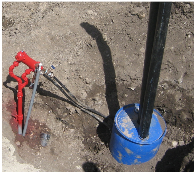
Figure 2.11: Heat Exchanger and Three-way Valve Enclosure. The three-way valve enclosure shown with the thermosiphon heat exchanger.
