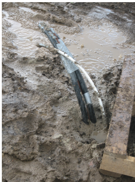
Figure 2.32: Vertical U-tube After Installation. This is the heavily monitored U-tube installed with a PEX pipe and thermocouples, before the horizontal pipes are connected. The U-tube is the two black pipes which are duct taped together and the PEX pipe is the smaller white pipe.
