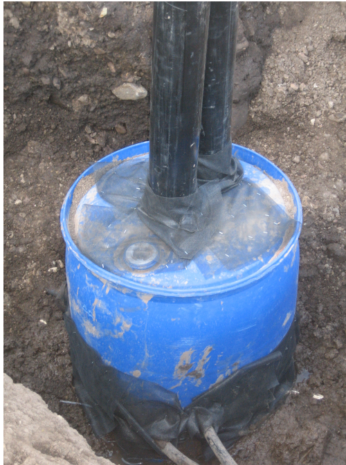
Figure 2.12: Valve Enclosure. Hardware cloth was stapled to the valve enclosure to keep soil and debris out after the enclosure was buried.
