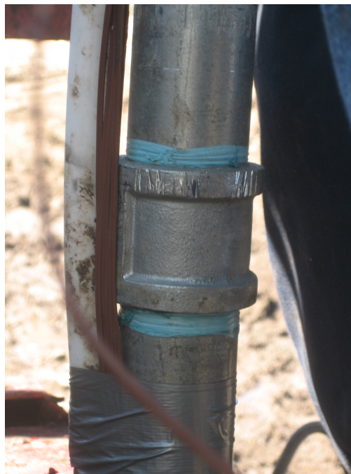
Figure 2.35: Thermosiphon Coupling. One of the NPT couplings on the thermosiphon pipe during installation, shown with a PEX pipe and thermocouples.
