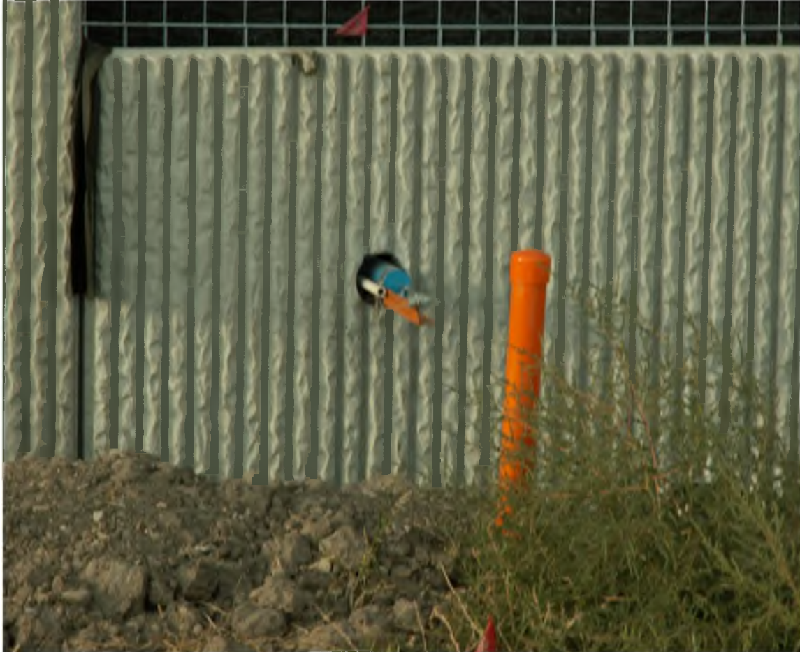
Figure 2-5. Horizontal inclinometer casing with pulley system perpendicular to the centerline alignment in this project.
