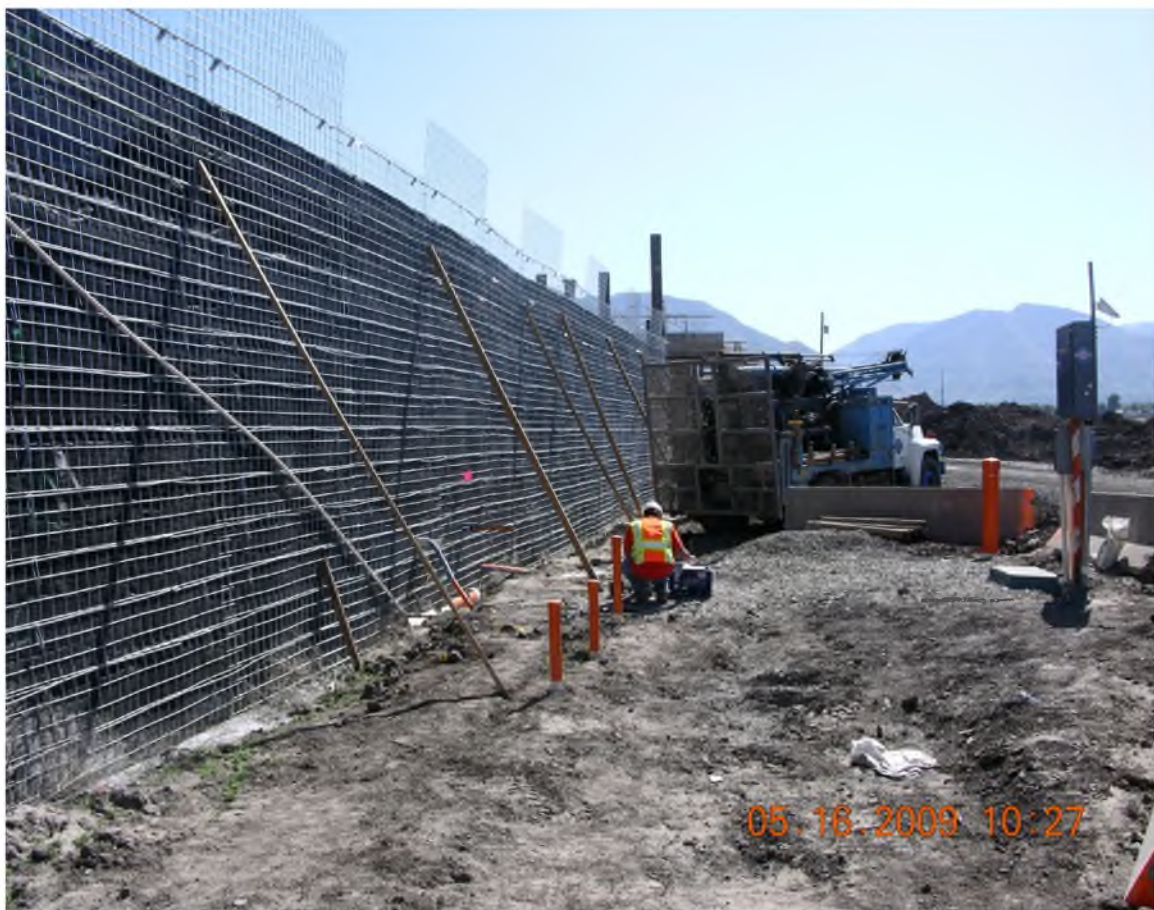
Figure 1-11. Outside view of MSE wall west of the bridge on the south side of SR 77 during construction. Location of the research instrumentation can be seen in the middle.
