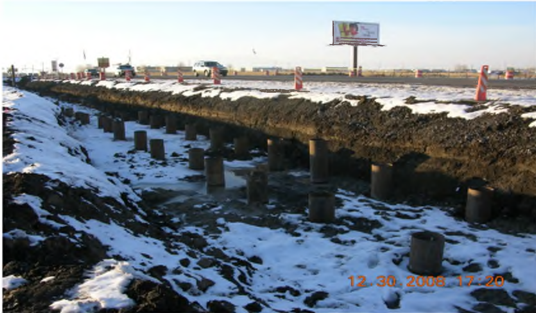
Figure 1-5. Steel pipe piles installed beneath MSE wall west of the bridge on the south side of SR77.
