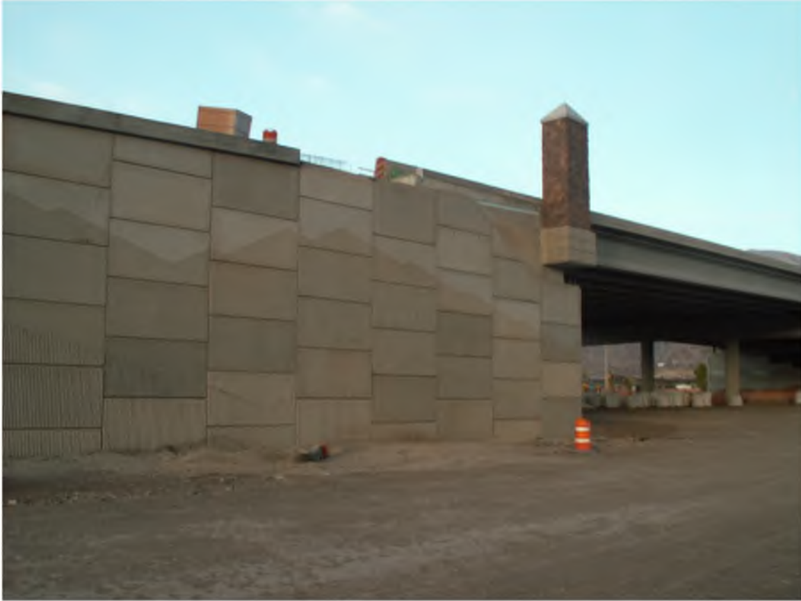
Figure 1-12. Completed MSE wall on the south side of the embankment west of the bridge.
