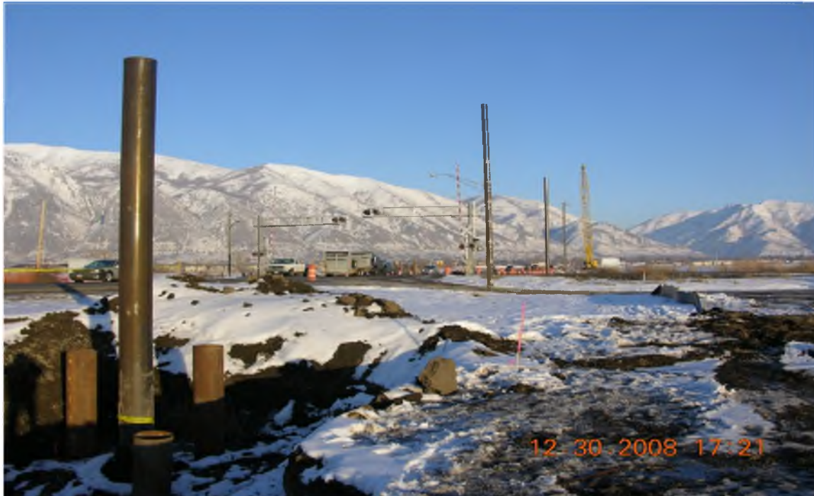
Figure 1-4. Initial stages of construction in December 2008 looking east. Piles for the west abutment can be seen in the left foreground. The railroad crossing can be seen in the middle.
