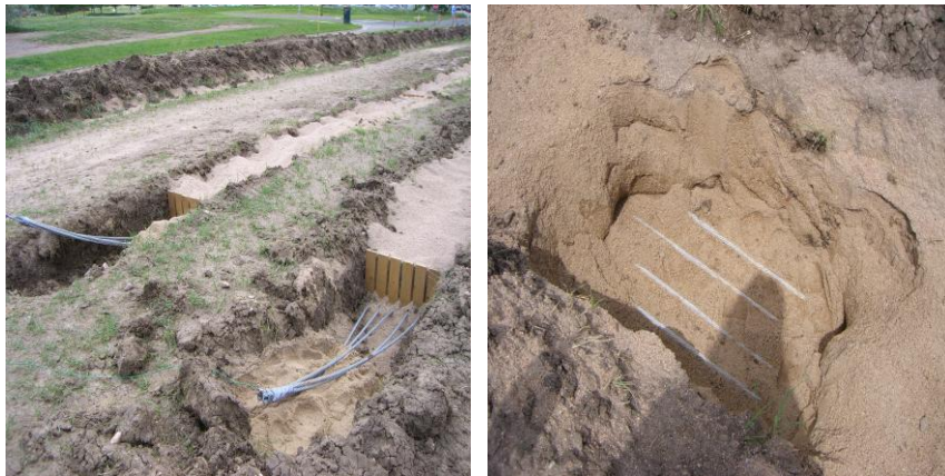
Fig. 11. (Left picture) Ends of two anchors extending from trenches 1 (left) and 2 (right), 7' apart. This shows the plywood spacers used to hold the strands approximately 4" apart in the trenches, as shown in the right photo. © 2009 IEEE. Reprinted, with permission, from 39.
