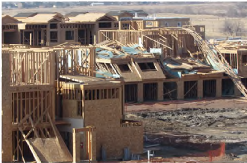
Figure 1.2: Damage sustained during the downslope windstorm of 1 December 2011 at a construction site near Station Park Mall in Farmington, UT. (Photo: John Horel)
